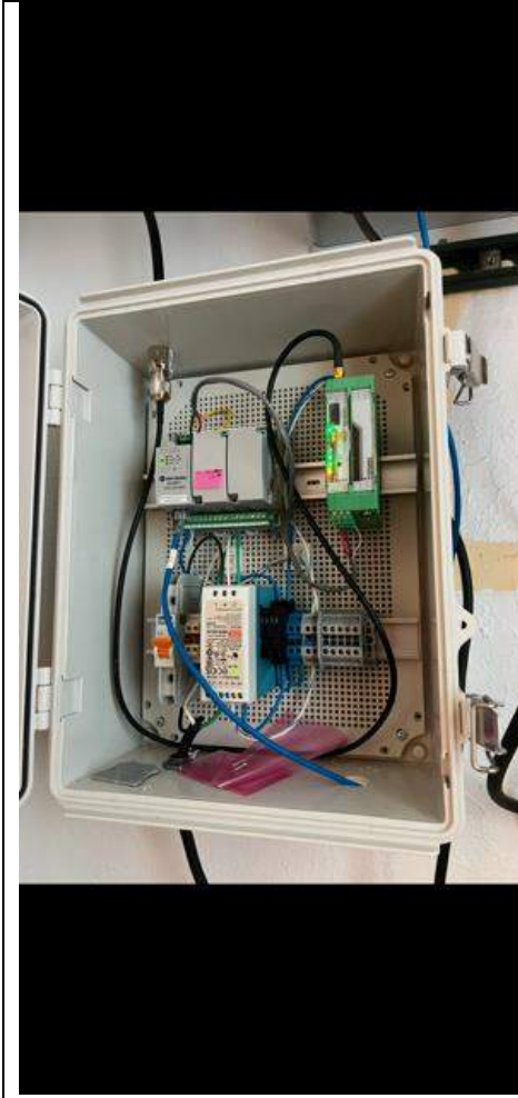
Figure 4.2 Micro820 PLC Panel
