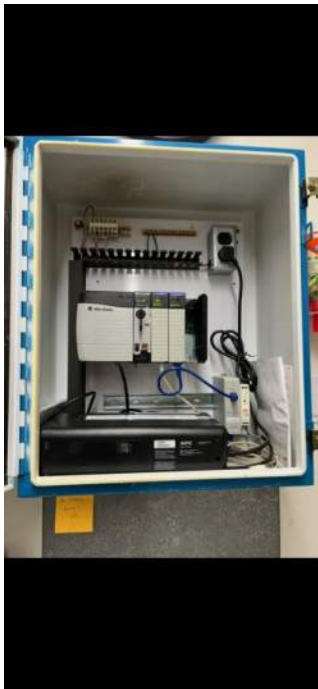
Figure 4.7 Nano/RO Main PLC Panel
