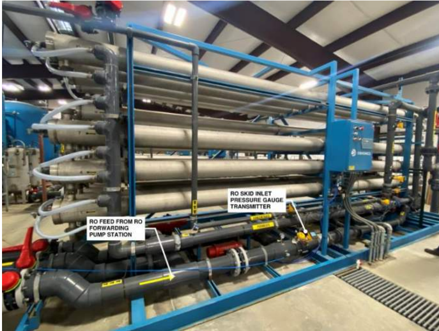
Figure 3.10 RO Skid Inlet Pressure Gauge Location
